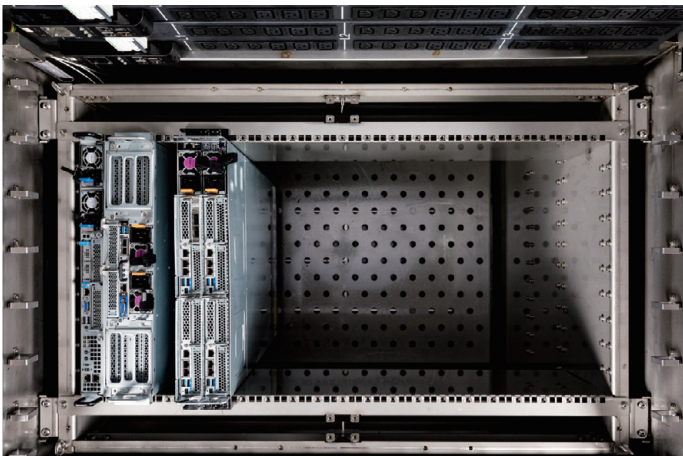
▲ Overhead view of A1P0-EB0 Tank
